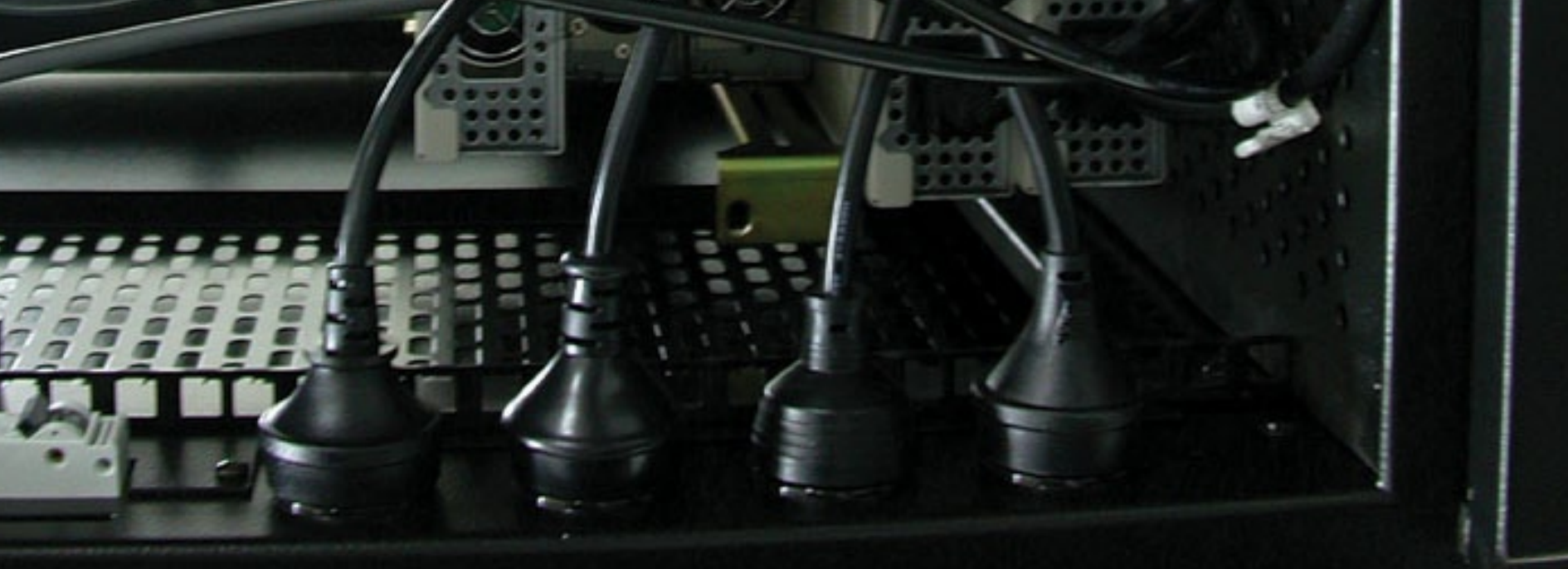
photograph of VA SERVER RACK by jesse reynolds (VA)
